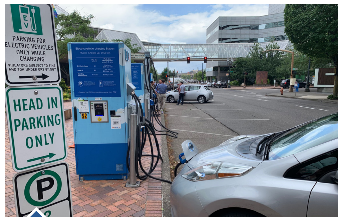
Electric vehicle charging stations make owning an EV more convenient.
